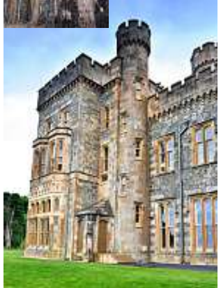
After: stonework was rebuilt in the large bay window which had to be completely taken apart to remove the rotting iron.
