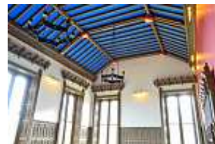
After: Think of the stories this dining room has still to tell, now that it has been brought back to its original condition.
