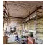
Before: water was dripping through the ceiling and running down the walls of the ballroom, before repairs began.
