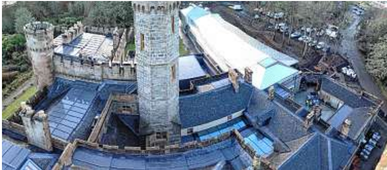
The complicated, leaking roof structure of the castle was one of the biggest challenges of the project. Picture: courtesy of Iain MacLeod
