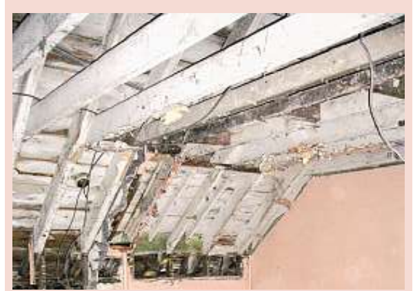
Lord Leverhulme preferred lots of fresh air while he was sleeping and the unusual roof structure found in his bedroom at Lews Castle showed it would have been open to the elements.
