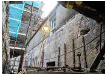
Putting the castle's own history on display, the 300-year-old walls of the original Seaforth Lodge were uncovered and form one of the features of the glass-roofed courtyard. Picture: courtesy of Iain MacLeod
