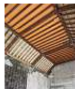
Before: the structure of the dining room roof was one of the most challenging areas to repair.
